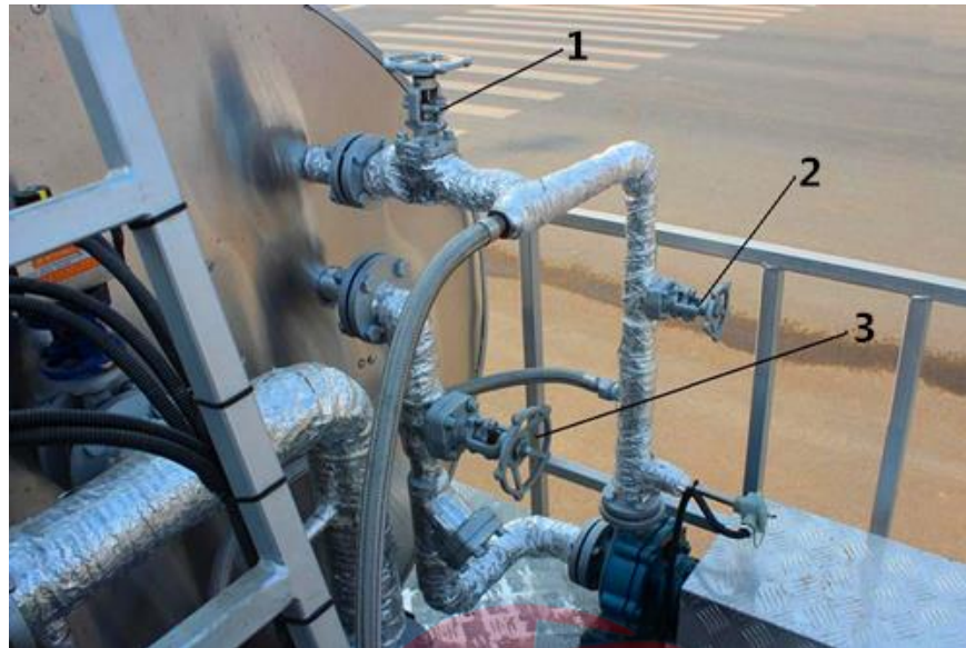
Fig. 11 Heat transfer oil valve
